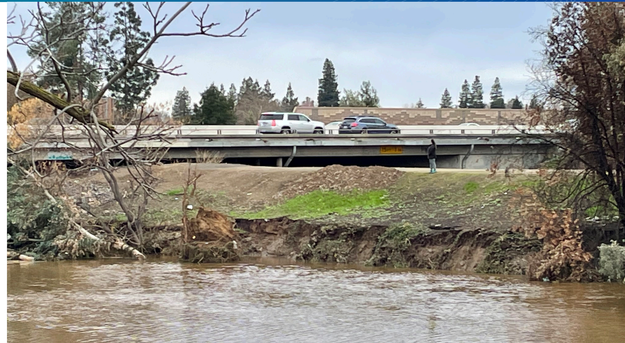
The Calaveras River levee was damaged during the January 2023 storms. The levee is one of many throughout Stockton that protect properties from flooding.
