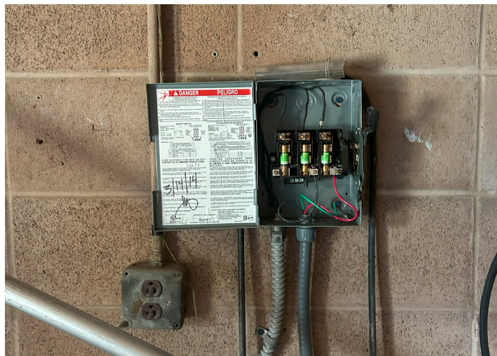
Image 29: Power for Pump Needing GFCI Protection
