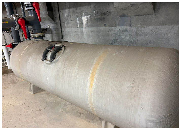
Image 44: Swimming Pool Filter Tank
