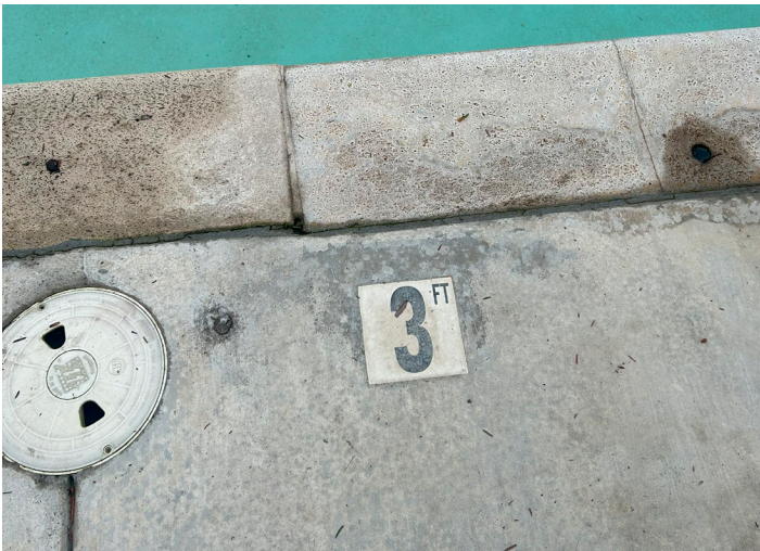
Image 7: Missing "No Diving" Marker at Swimming Pool
