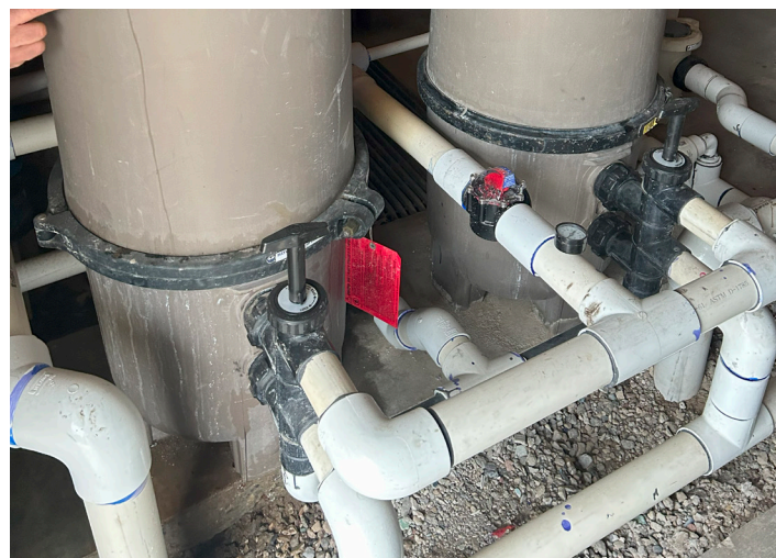
Image 33: Concrete Missing By Filters
