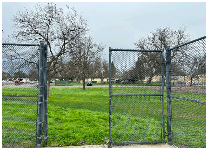
Image 36: Non-Code Compliant Gate
