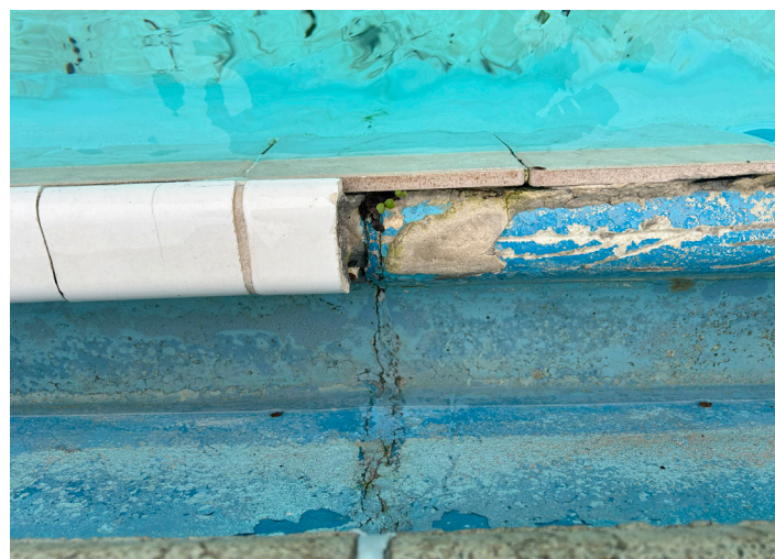
Image 47: Missing Tile in Swimming Pool
