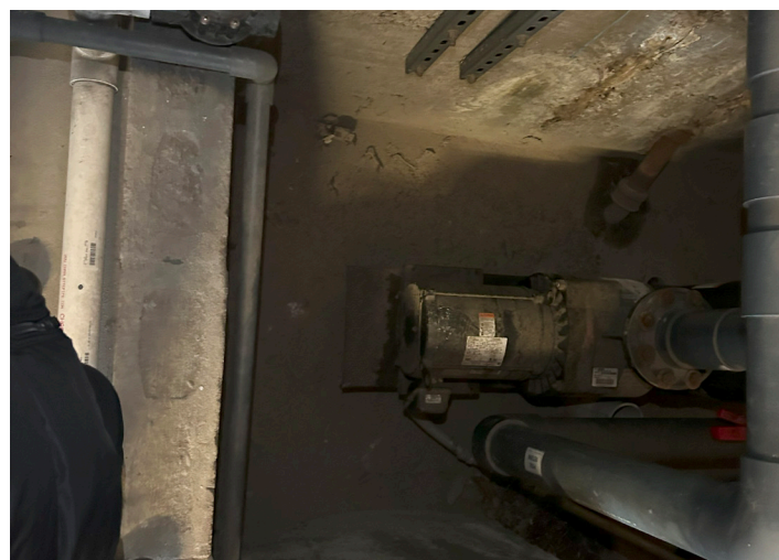
Image 31: Piping Missing Directional Flow Labeling
