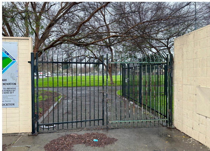
Image 45: Non-Code Compliant Gate
