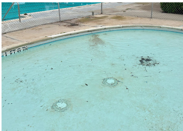
Image 27: Failing Wading Pool Finish
