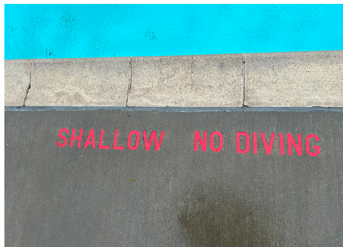
Image 49: Missing "No Diving" Graphic Marker
