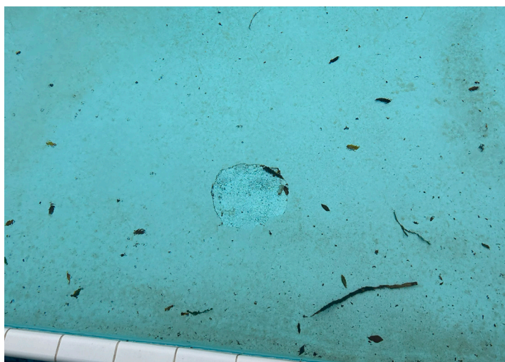
Image 46: Missing Plaster in Swimming Pool
