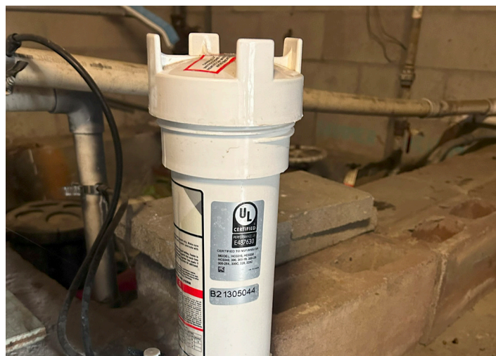
Image 14: Chlorine Tablet Feeder for Wading Pool
