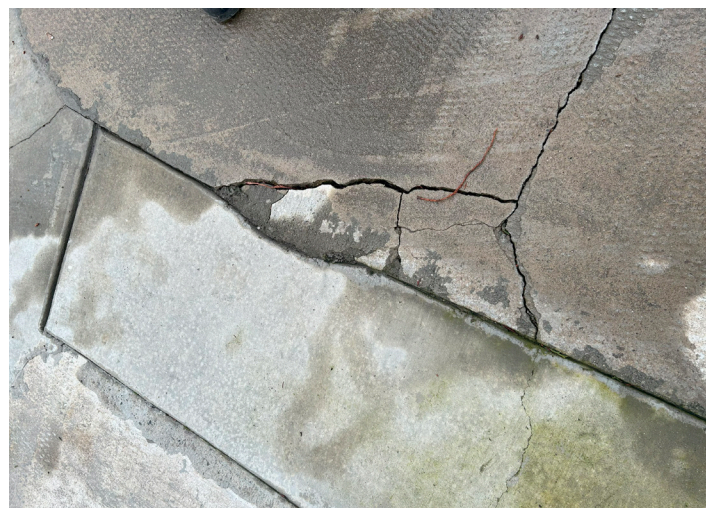
Image 6: Failing Pool Deck
