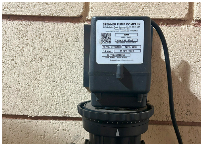
Image 5: Chlorine Metering Pump for Swimming Pool
