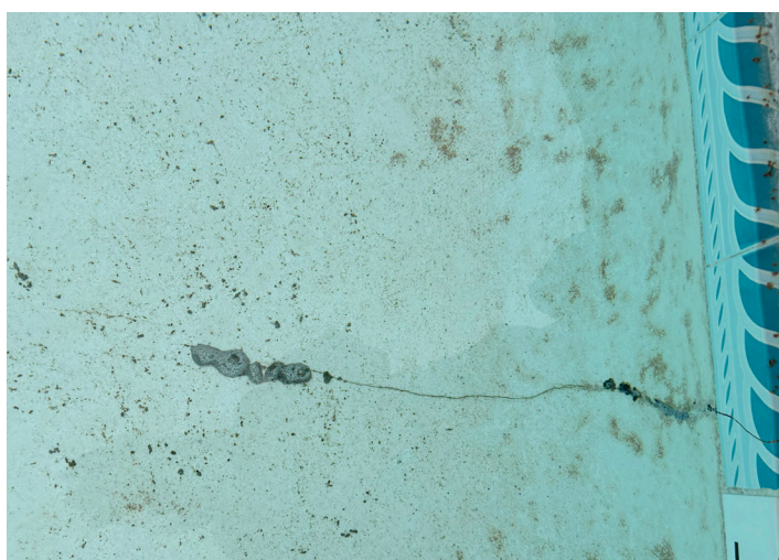
Image 21: Cracked Plaster in Wading Pool
