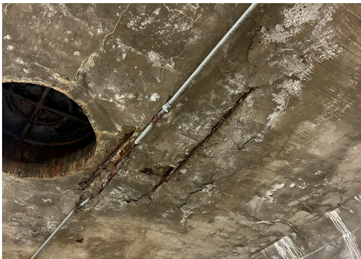
Image 41: Failing Ceiling in Mechanical Room
