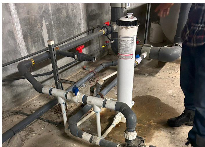
Image 37: Chlorine Tablet Feeder for Swimming Pool
