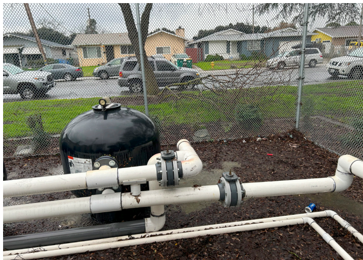
Image 50: Piping Missing Directional Flow Labeling
