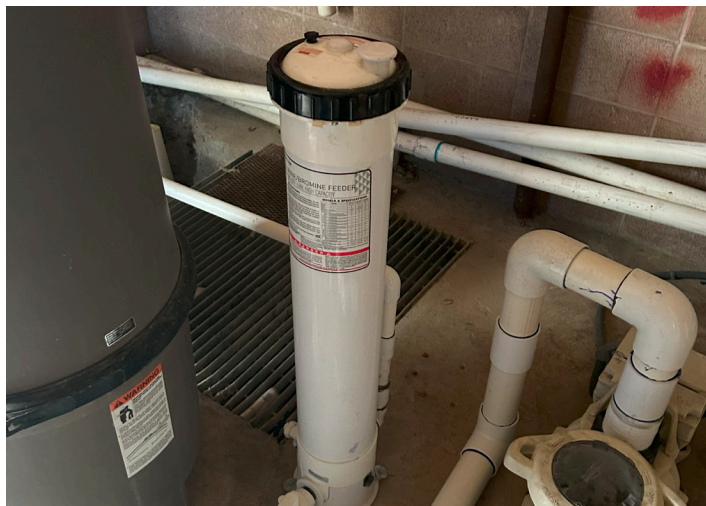
Image 28: Chlorine Tablet Feeder for Swimming Pool
