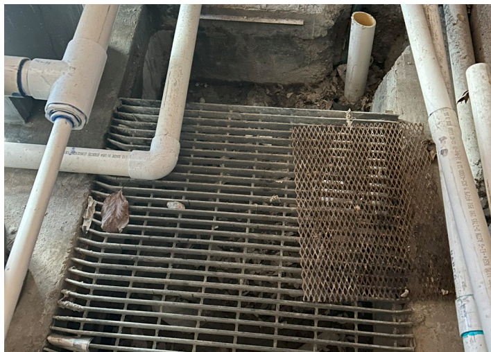
Image 34: Concrete Missing Behind Filters
