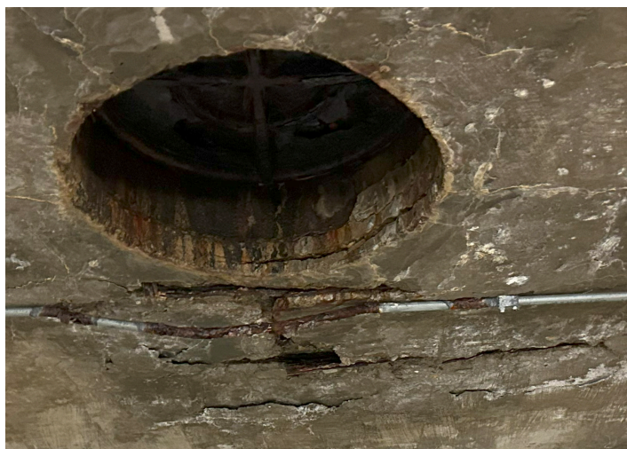
Image 39: Failing Ceiling in Mechanical Room
