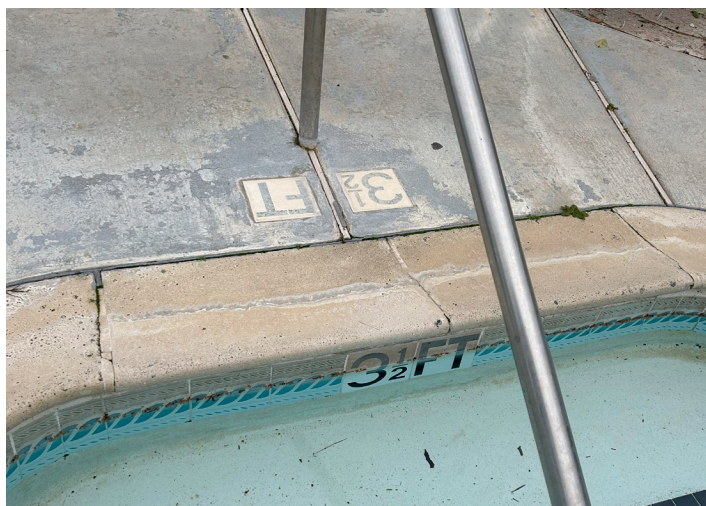
Image 19: Missing "No Diving" Marker at Swimming Pool
