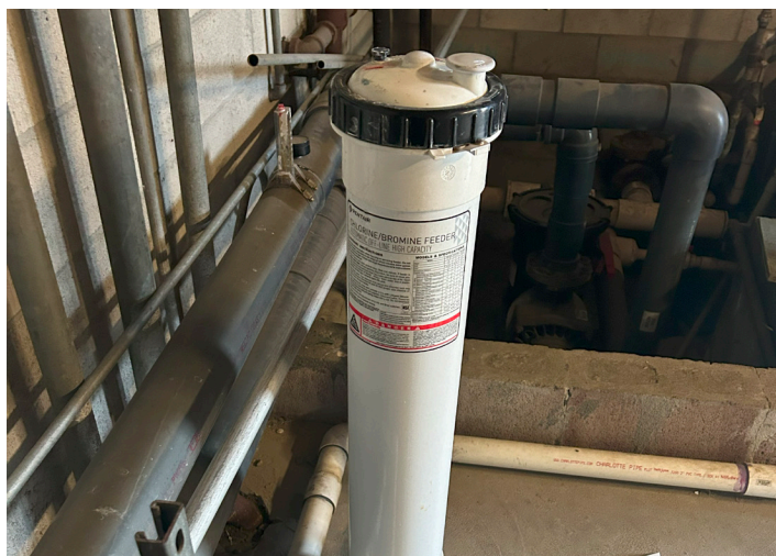
Image 13: Chlorine Tablet Feeder for Swimming Pool
