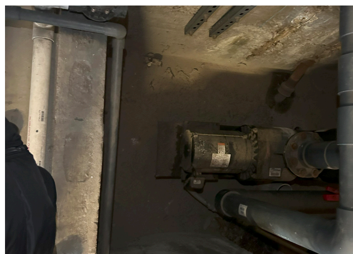
Image 22: Poor Access to Pump Pit
