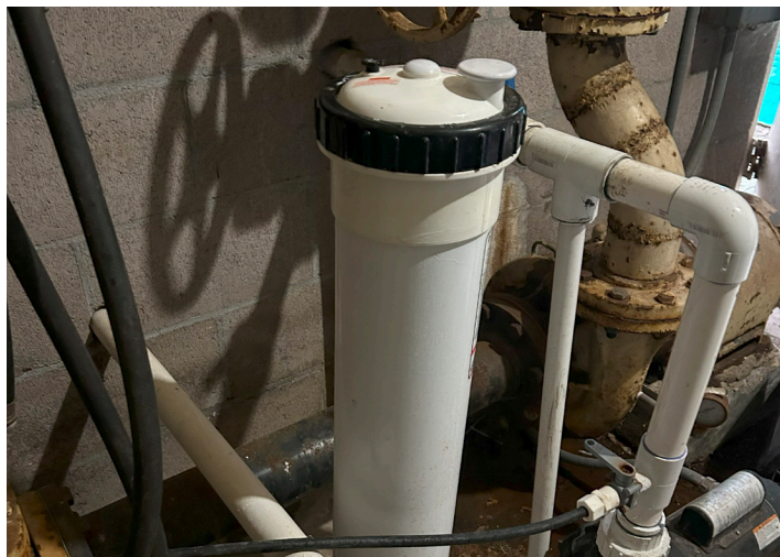
Image 44: Chlorine Tablet Feeder for Swimming Pool
