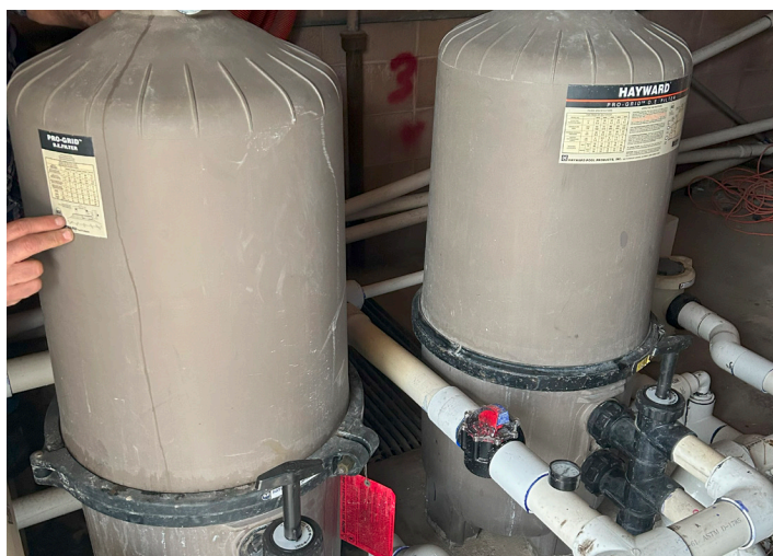
Image 30: DE Filter Tanks
