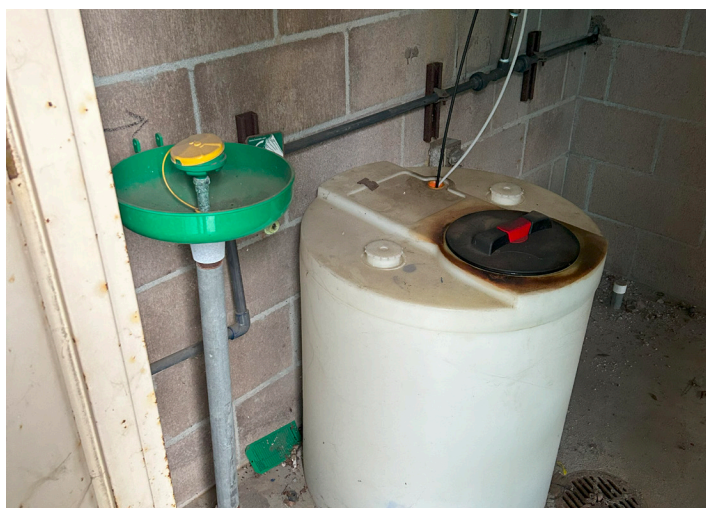
Image 52: Abandoned Chemical Equipment
