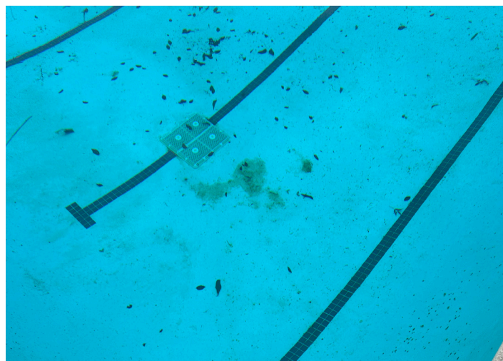
Image 20: Stained Plaster in Swimming Pool
