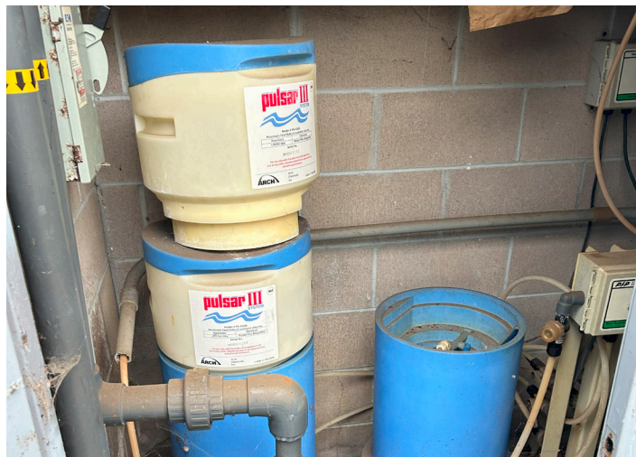
Image 51: Abandoned Chemical Equipment
