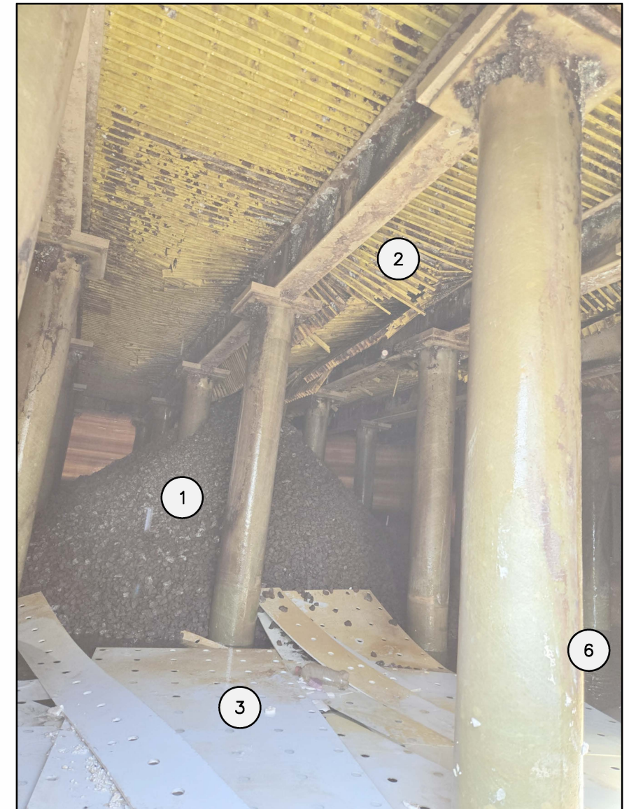
INSIDE VIEW OF BIOSCRUBBER FROM SIDE MANWAY
