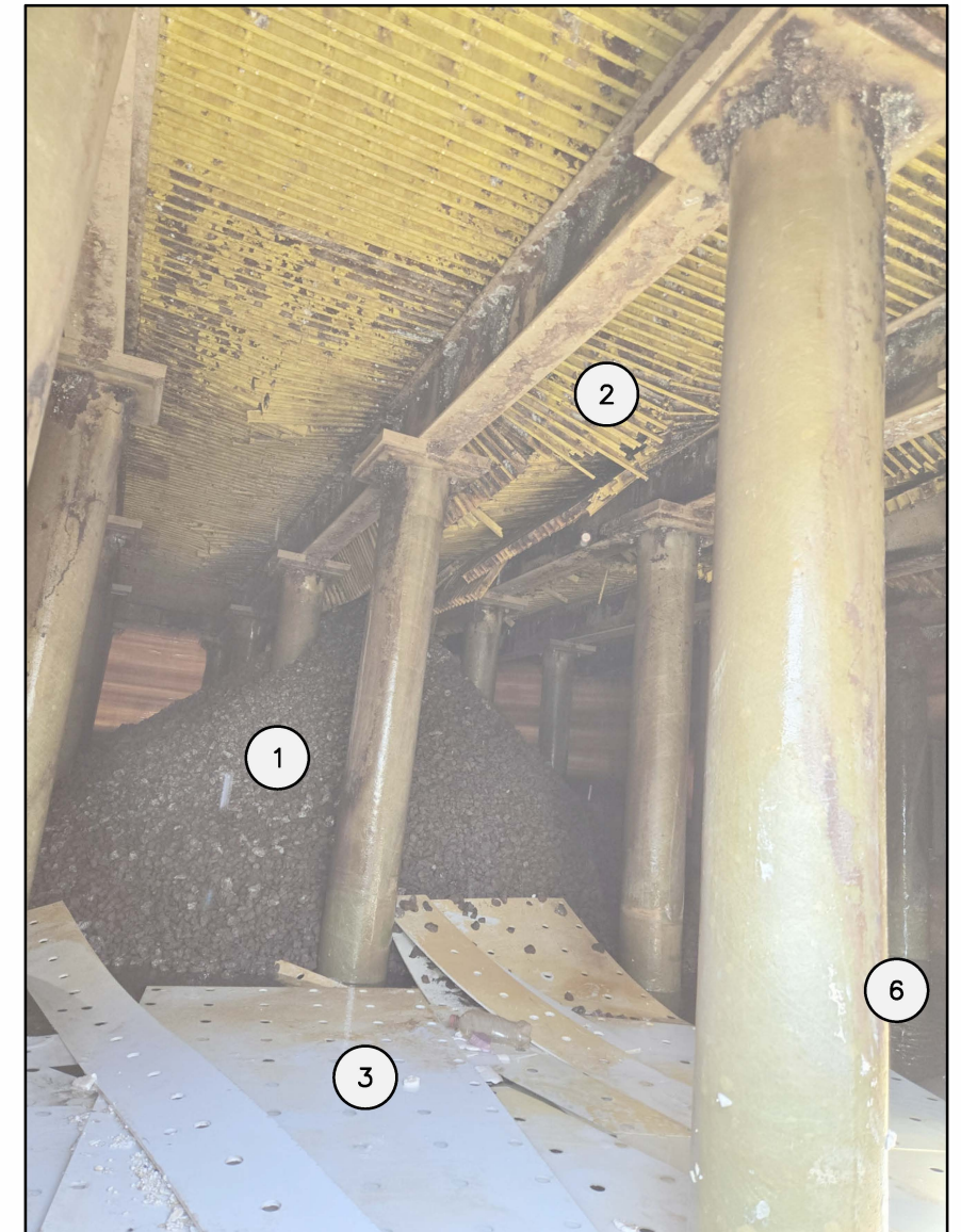
INSIDE VIEW OF BIOSCRUBBER FROM SIDE MANWAY
