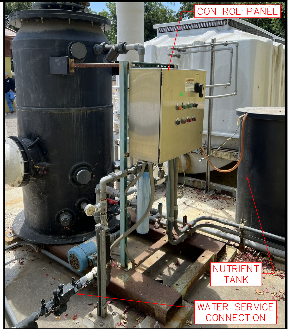
PHOTO 5 - EXISTING CONTROL PANEL
