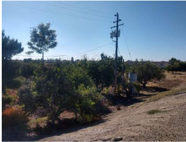
Figure 17 – View of transformers adjacent north near levy.
