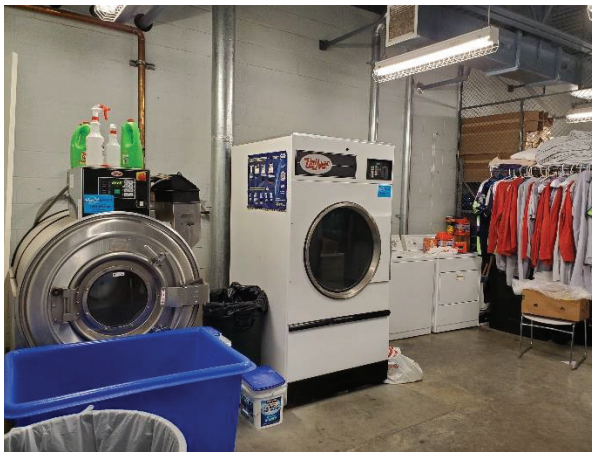
SECTION 3.5: TEAM LAUNDRY FACILITY
