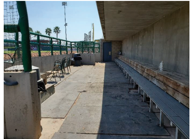
SECTION 7.5: THE DUGOUT HAS ANTI-SKID FLOORING BUT THE RUBBER MATS ARE LOOSE WITH GAPS AND PRESENT A TRIPPING HAZARD.
