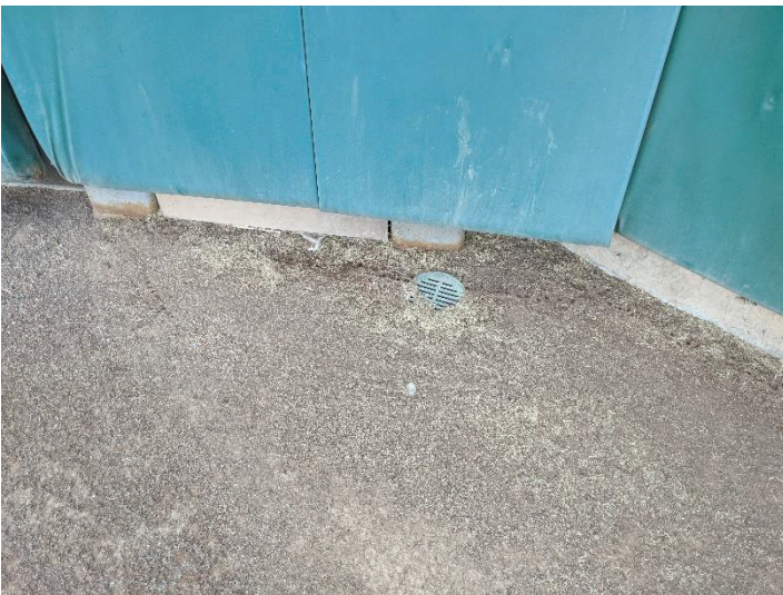
SECTION 7 (PLAYING FIELD) SURFACE DRAINS INSTALLED ON WARNING TRACK ARE NOT LEVEL WITH WARNING TRACK
