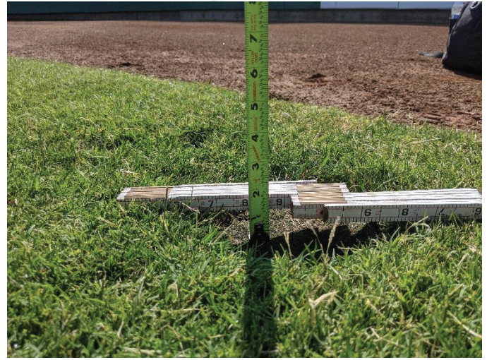
SECTION 7 (PLAYING FIELD) – VALVE BOX IS INSTALLED TOO LOW
