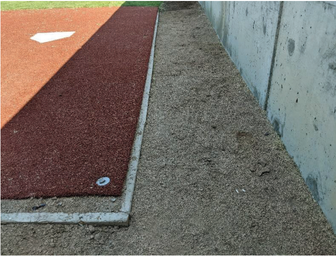
SECTION 7 (PLAYING FIELD) – ADD ADDITIONAL MATERIAL AROUND WOOD CURB in BULLPEN– TRIPPING HAZARD
